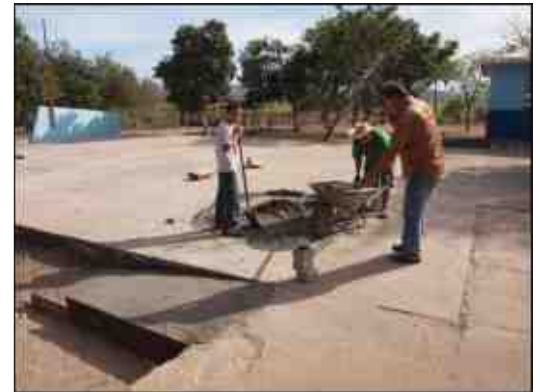
The school provided cement and other materials, and parents, teachers and older pupils provided the labor.
