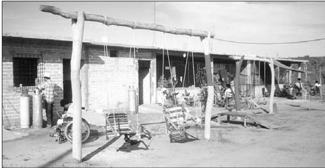
All the buildings seen here were built during the last year as part of the new PROJIMO Rehabilitation Center in the village of Coyotitan. Construction is still in process.
